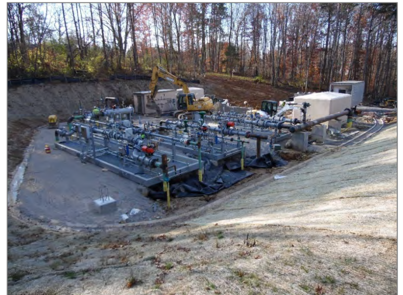
Gate Station Commissioning December 2018
