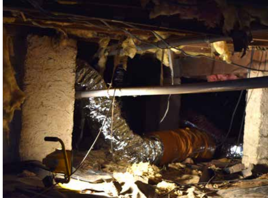
Above: Through KUB's low-income weatherization programs, problems like damaged ductwork and insulation are remedied, making homes more efficient and lowering energy bills.
