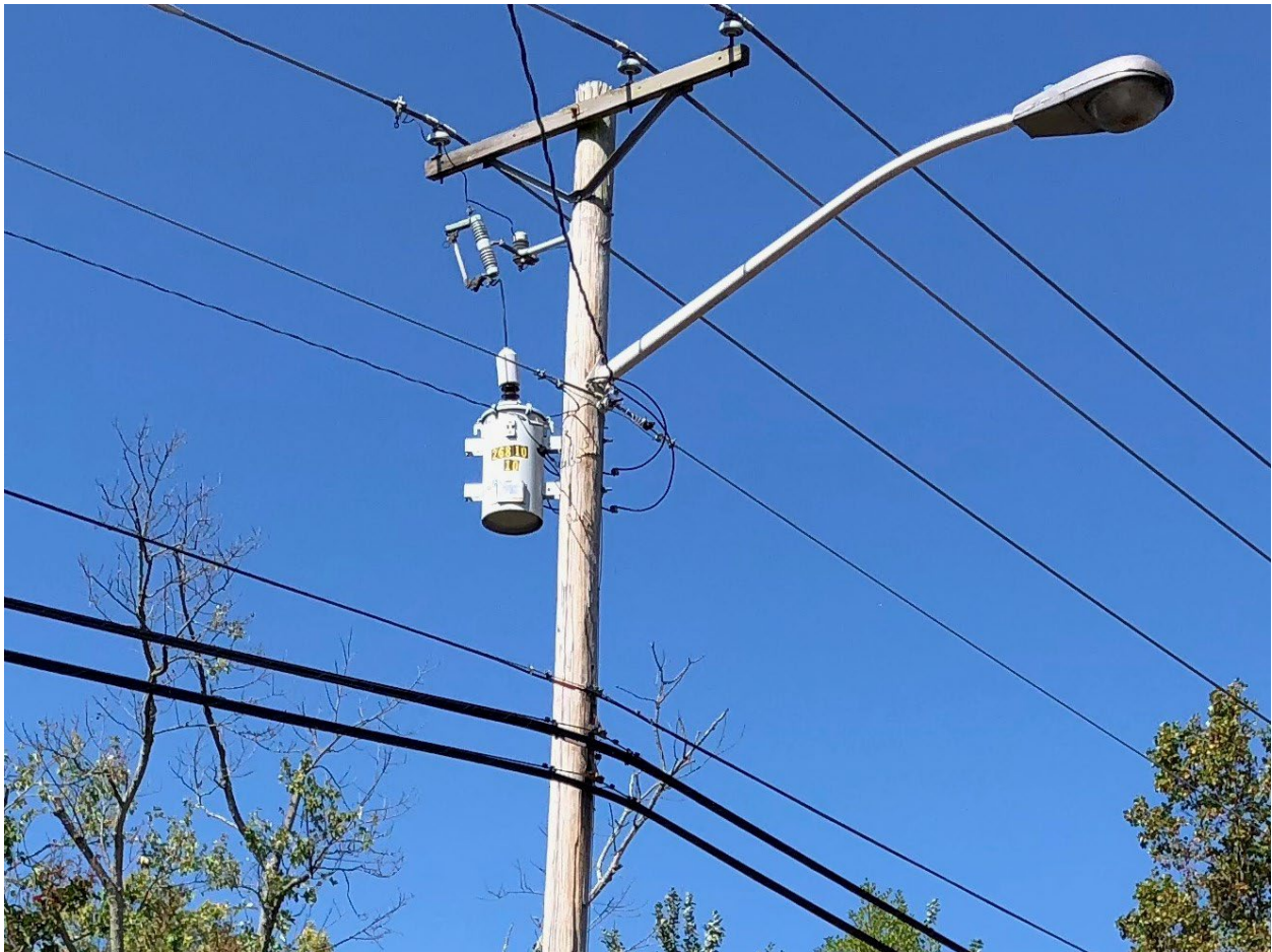
Figure 4.1 Typical KUB Pole with Multiple Users Attached
