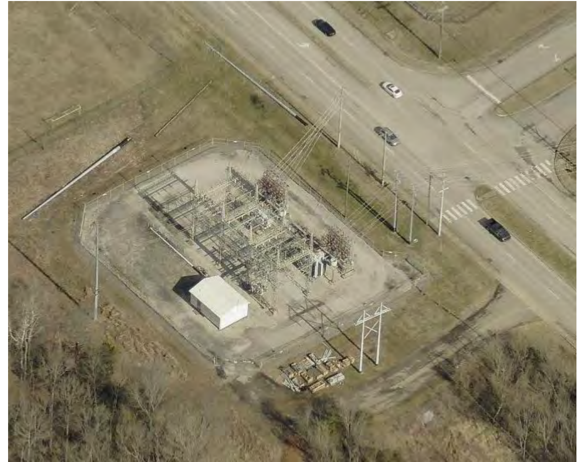
Dry Gap Substation
