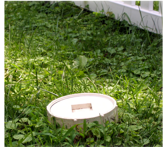
Sewer lateral cleanout cap
