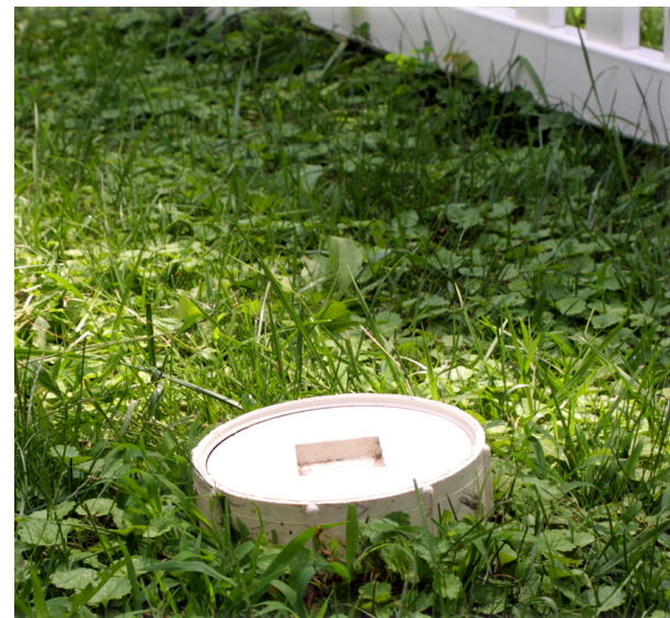
Sewer lateral cleanout cap
