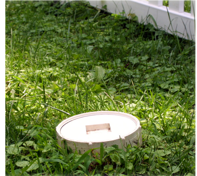
Sewer lateral cleanout cap
